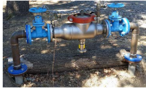
Example of a backflow prevention assembly
