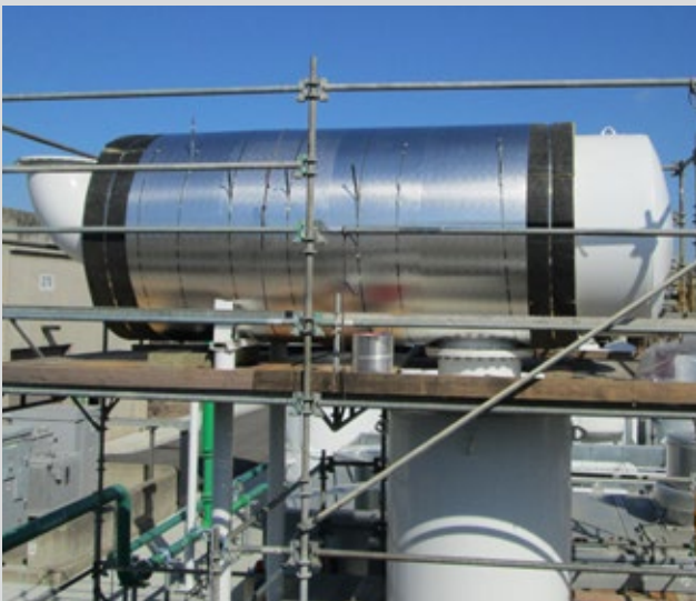
A horizontal silencer was installed at the SEP Oxygen Generation Plant for noise remediation.
