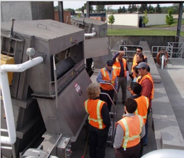
SEP Headworks project team visits Willow Lake Water Pollution Control Facility (Oregon) to discuss lessons learned around Grit Handling technology.
