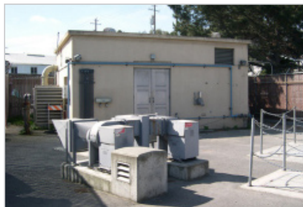
Figure I-5. Mariposa Pump Station
