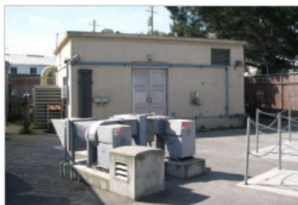
Figure I-5. Mariposa Pump Station
