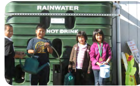
Longfellow Elementary's Rainwater Harvesting System
