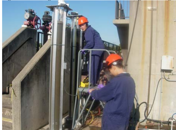
Figure 1. Settling columns installed at SEP during the testing event.
