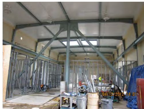
Interior seismic and tenant improvement work at the Lake Merced existing pump station building
