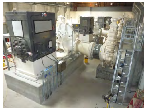
Mechanical pump arrangement inside the new LMPS building
